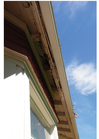
Dry rot at eave
