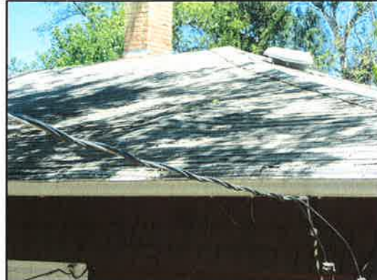
Hump in Roof
