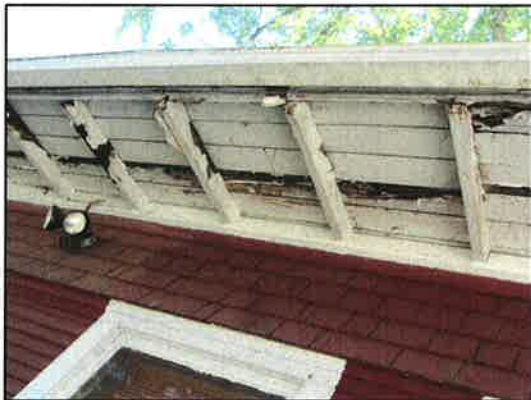
Water Damaged Soffit Boards
