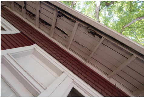
Dry rot at Eave
