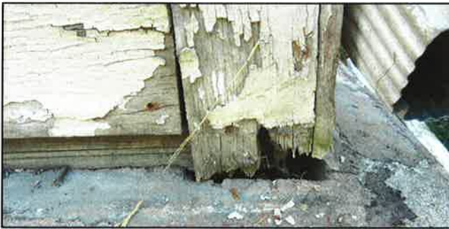
Rotted Porch Columns
