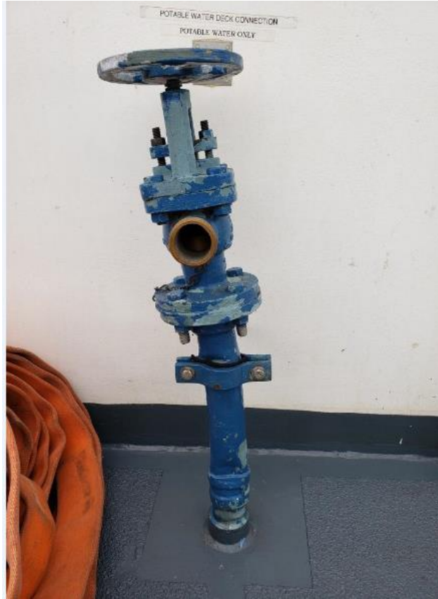
FIGURE 1. PHOTO OF DAMAGED DECK FILL VALVE & PIPING
