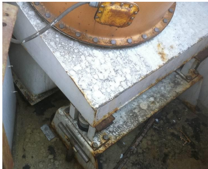
FIGURE 3: VIBRATION ISOLATING MOUNTS ON CGC STURGEON BAY
