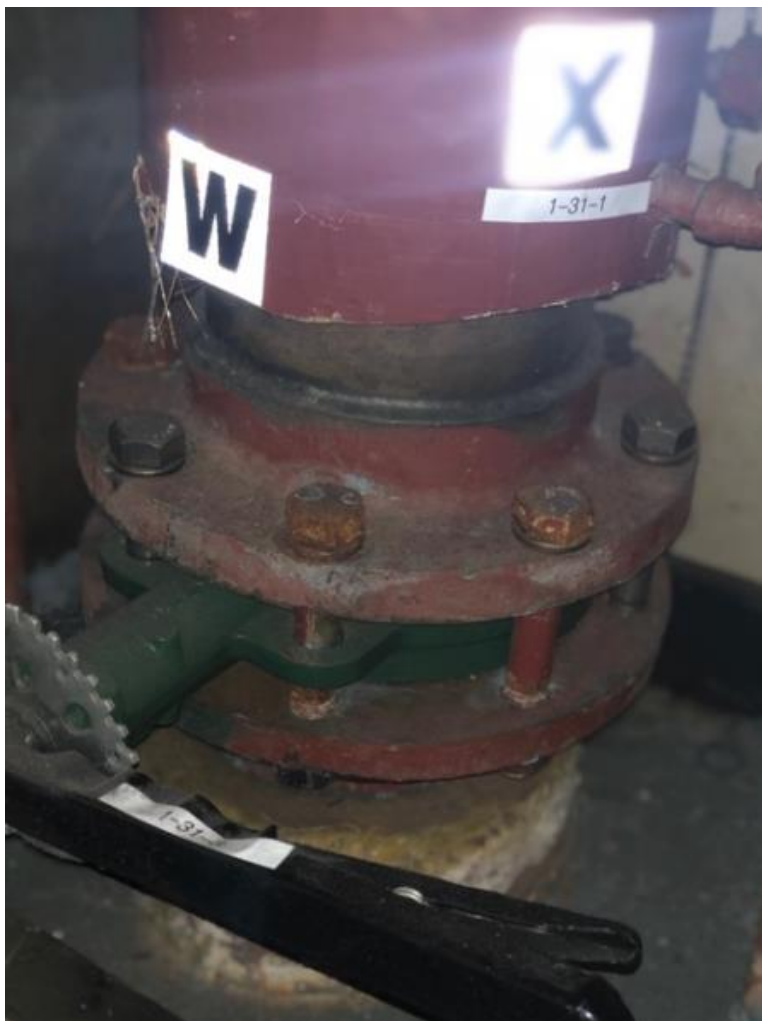
FIGURE 1. PHOTO OF AFFECTED FIREMAIN VALVE
