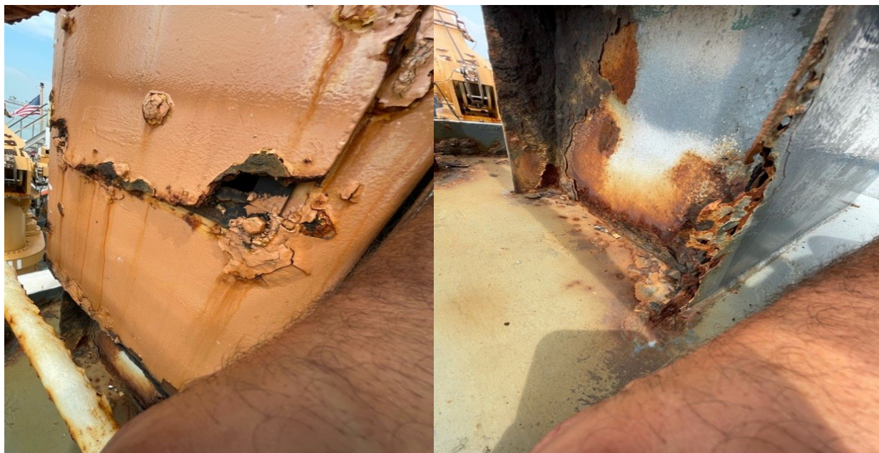
PHOTO 1: SMALL BOAT DAVIT CONSOLE FOUNDATION, WASTED METAL
