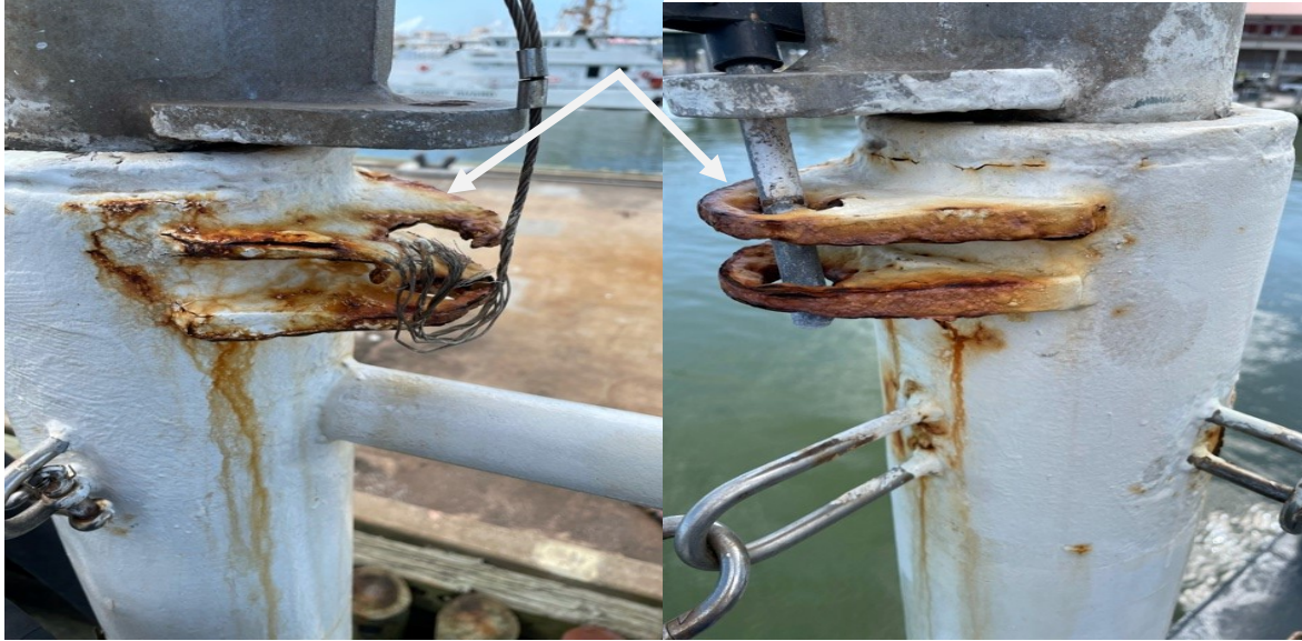
PHOTO 1: PORTABLE HOISTS BRACKETS, RENEW
