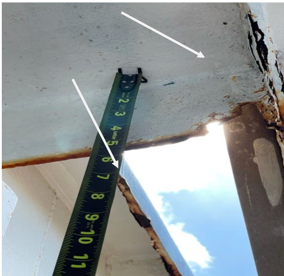
PHOTO 1: BUOY-DECK BEAM, PORT SIDE
