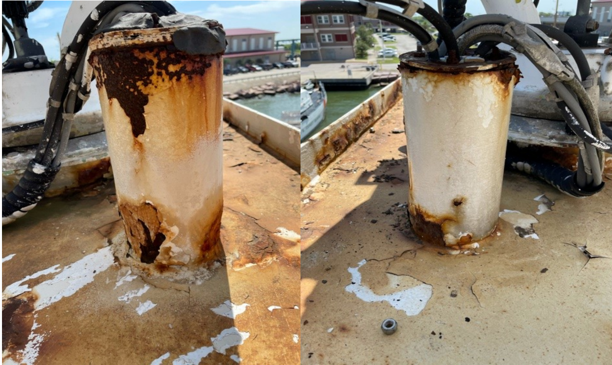
PHOTO 1: STUFFING TUBES CONDITIONS
