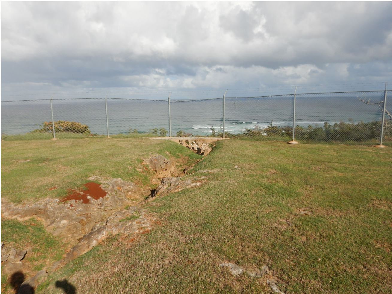
1 2 Figure 3.1-4 Drainage Swale Worn Down to Limestone with Limited Vegetation
