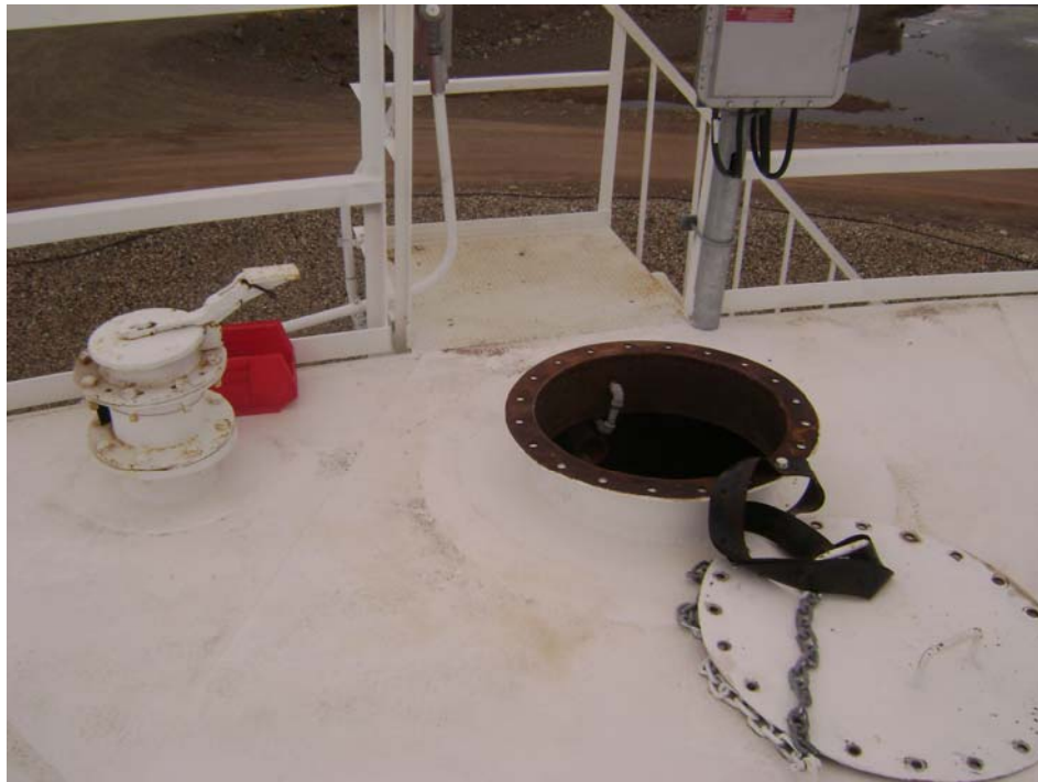
10" Thief Hatch with ITT Barton ATG Probe Assembly and 24" Manway
