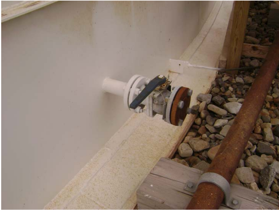
2" with ¼ Turn Ball Valve in Dead Shell (Typical of 2) and Tab with Ground Wire (Note: Ball valve used for leak detection in interstitial space.)
