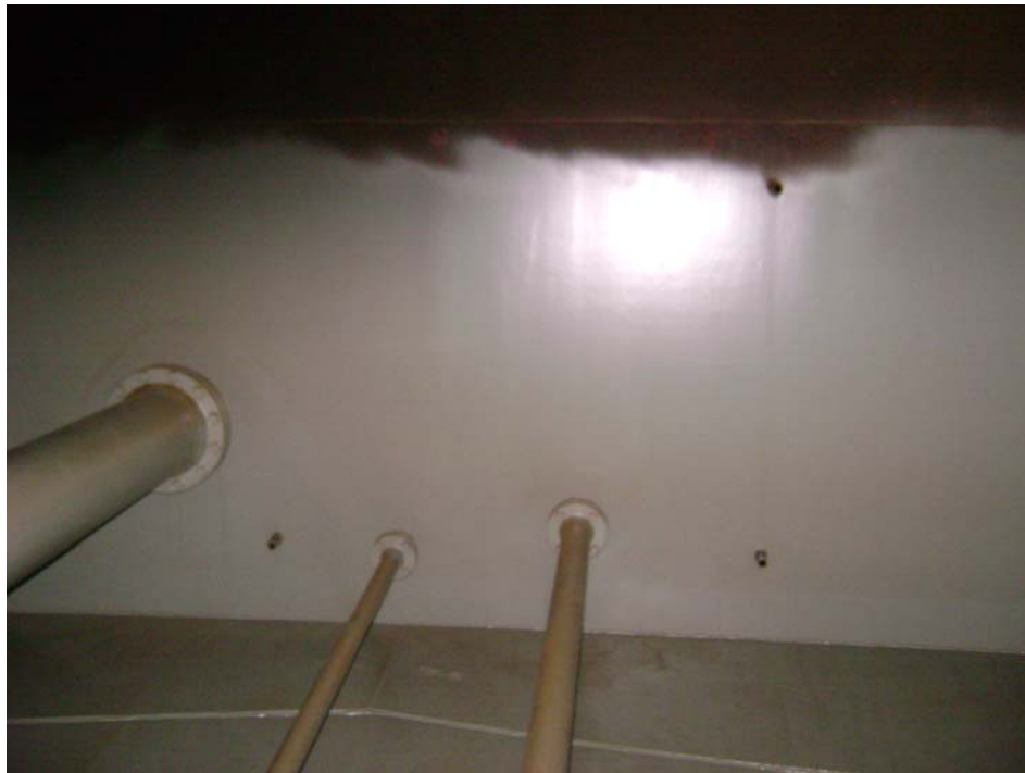
Left to Right: 12" Fill Nozzle, 1" Thermal Relief Nozzle, 2" Water Draw-Off, 3" Low Fuel and Abandoned Nozzles for Low Level Alarm
