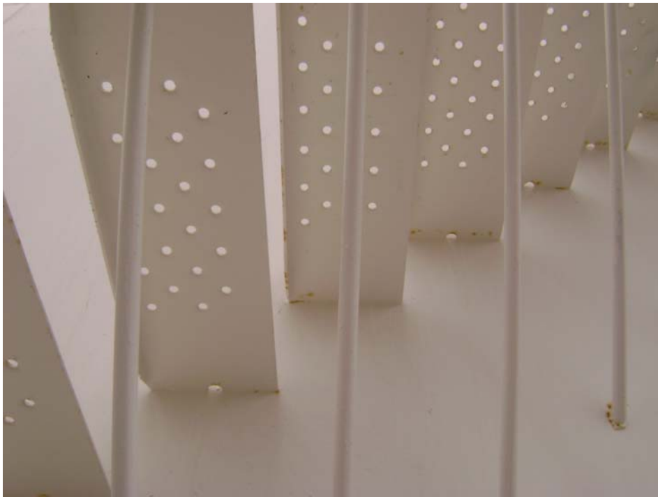
Spiral Stairs (Note: Minor coating failure and corrosion.)
