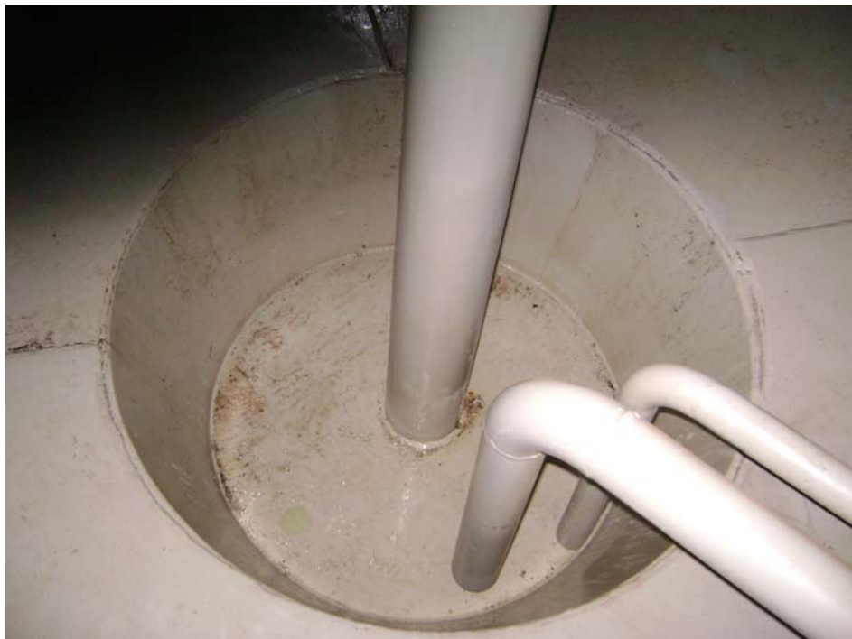
Left to Right: Center Roof Support Column, 3" Low Fuel Piping and 2" Water Draw-Off Piping in Center Sump
