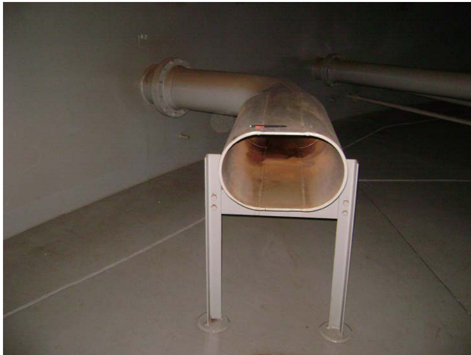
12" Fill Piping with Diffuser
