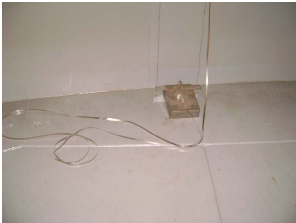
Float for Shand & Jurs Tape Gauge (Note: Tape was not functional.)
