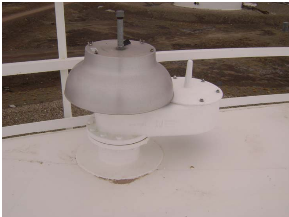
Shand & Jurs Pressure/Vacuum Vent (Typical of 2)
