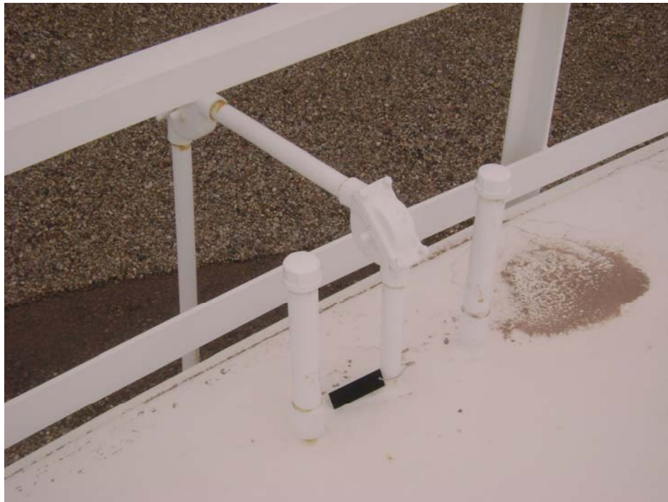
Penetrations for Shand & Jurs Tape Gauge Float and Guide Wires
