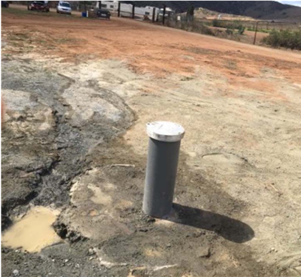
Figure 2-4 Brown Field BPS Well Sealed and Capped
