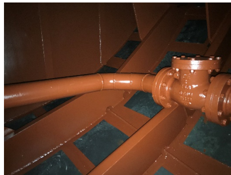
Continuation of piping in Void 3-78-2
