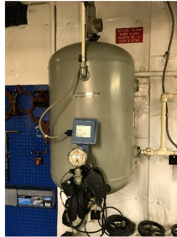
Fuel Shutdown Air Receiver
