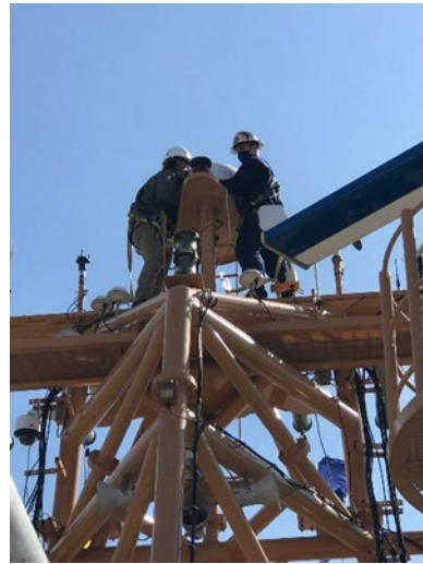
Bigelow Antenna in service
