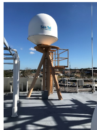
Ku-Band Antenna Mast
