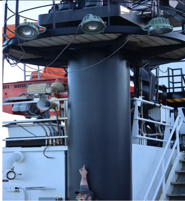
Position of new camera – Port side Crane Tower:
