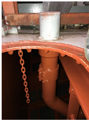
Pipe penetrating deck into Oceo Winch Room
