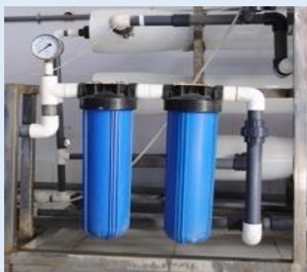
Sediment cartridge filters (1 micron) installed at the factory for fine filtration
