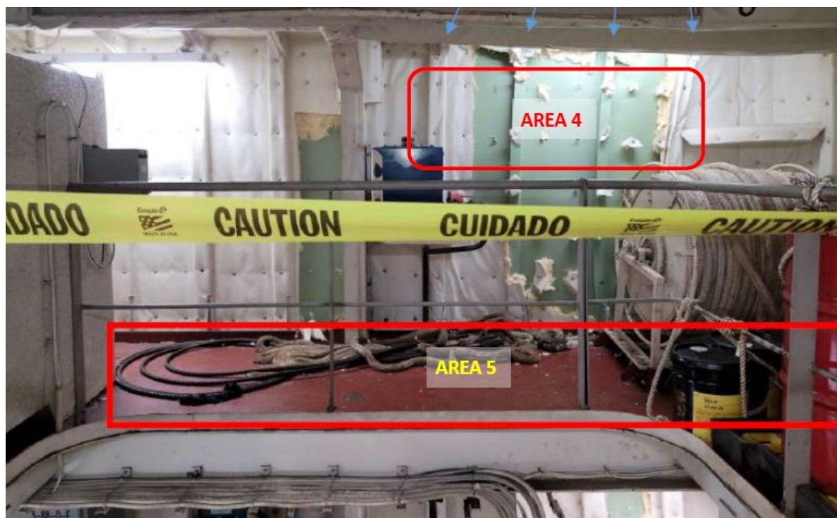
PHOTO 3. REPAIR AREAS 4 & 5, TRANSOM STIFFENERS & MAIN DECK, PROPULSION THRUSTER ROOM UPPER LEVEL (LKG AFT)
