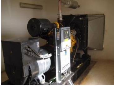
Vault A: Emergency stand-by generator well maintained.
