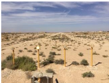
R/W 31 Approach lights operational. Some need new lamps.
