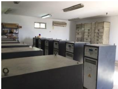
Vault A: CCRs and MDP in good working condition.
