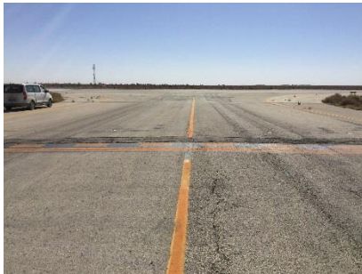
Taxiway Lima 4 Stop-Bar for Runway 26
