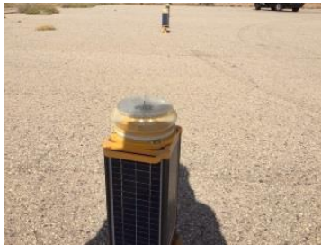
R/W 13 Solar lighting operational.
