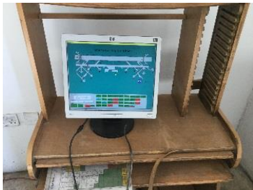
Vault A: Remote Control/Mimic Panel for local control is operational.
