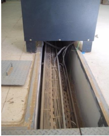
Vault B: Airfield lighting cables in good condition.
