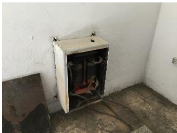
Vault A: R/W 31 Approach Lighting Sequenced Flashing Light transformer is burnt and needs replacing.
