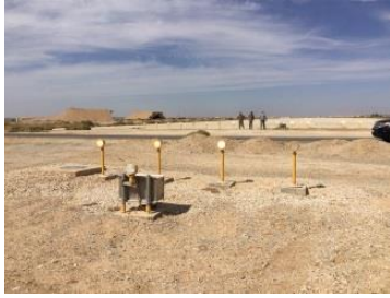
R/W 31 Sequenced Flashing Light not operational.
