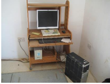
Vault B: Remote Control/Mimic Panel for local control is not operational.
