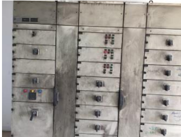
Vault A: MDP in good working condition, but needs good surface cleaning.
