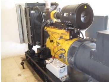
Vault B: Emergency stand-by generator well maintained and operational.
