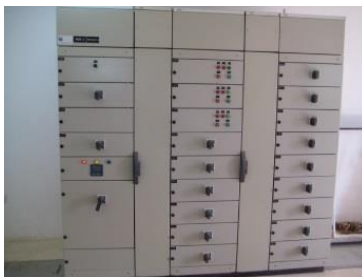
Vault B: MDP operational and in good working condition.
