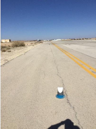
Taxiway Lima 4, Solar Taxiway Edge Light supplementing missing permanent light fixture.
