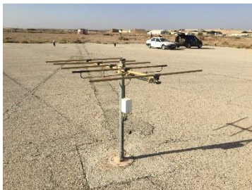
R/W 13 Solar lighting RF Antenna not operational.
