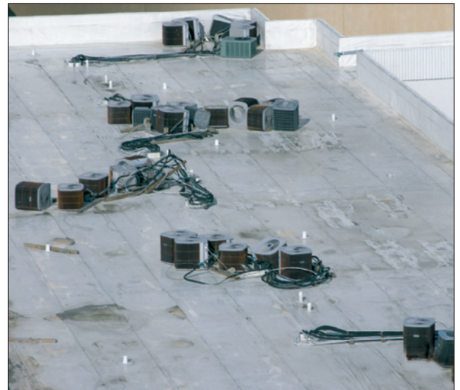
Figure 6. Sleeper-mounted condensers displaced by high winds.
