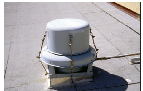
Figure 4. To overcome blow-off of the fan cowling, this cowling was attached to the curb with cables.
