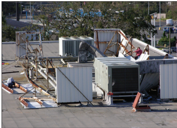
Figure 9. Several of the equipment screen panels were blown away. Loose panels can break glazing and puncture roof membranes.
