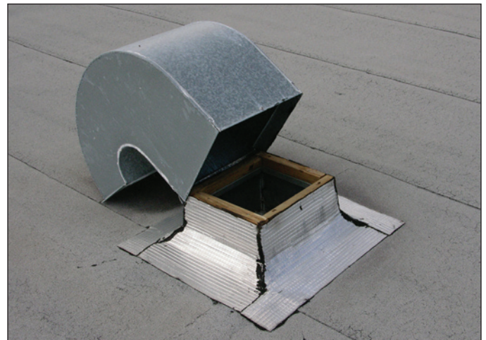
Figure 1. This gooseneck was attached with only two small screws. A substantial amount of water was able to enter the building during the hurricane.
