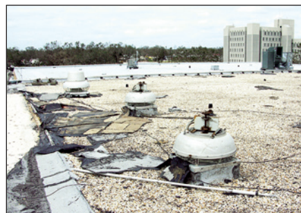
Figure 3. Cowlings blew off two of the three fans shown in this photo. Cowlings can tear roof membranes and break glazing.
