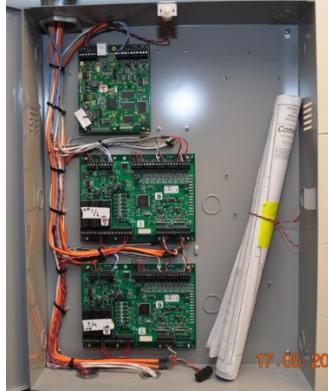
Main Control Boards
