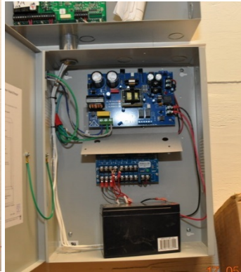
Main Control Battery Supply
