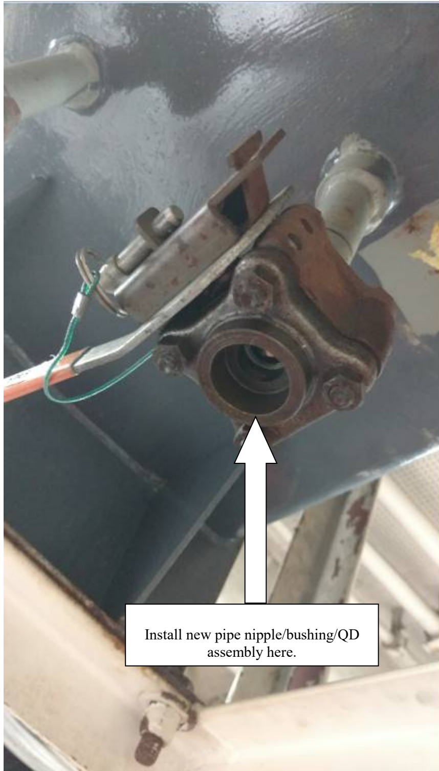
FIGURE 3. PHOTO - TYPICAL HEAD TANK DRAIN VALVE
