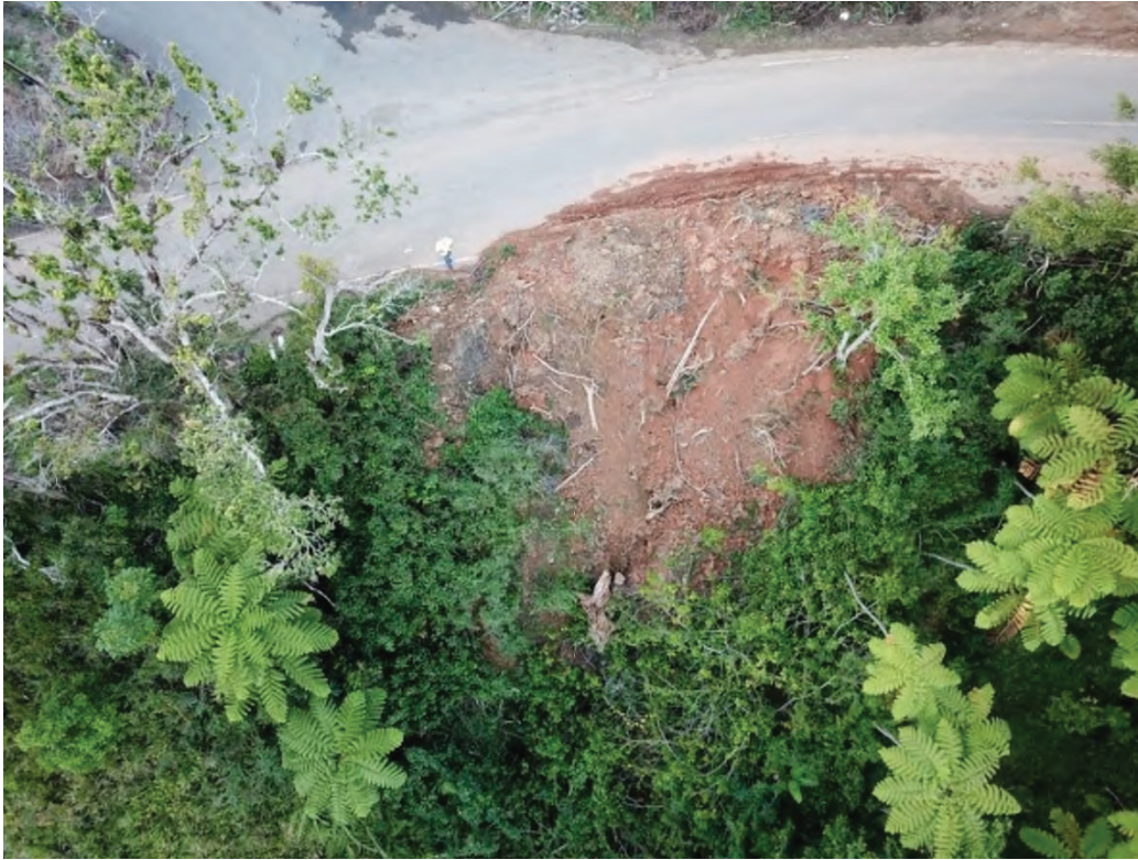
Figure 4: Top View of the Landslide Located at PR 179 Km 13.25 (Photo Supplied)
