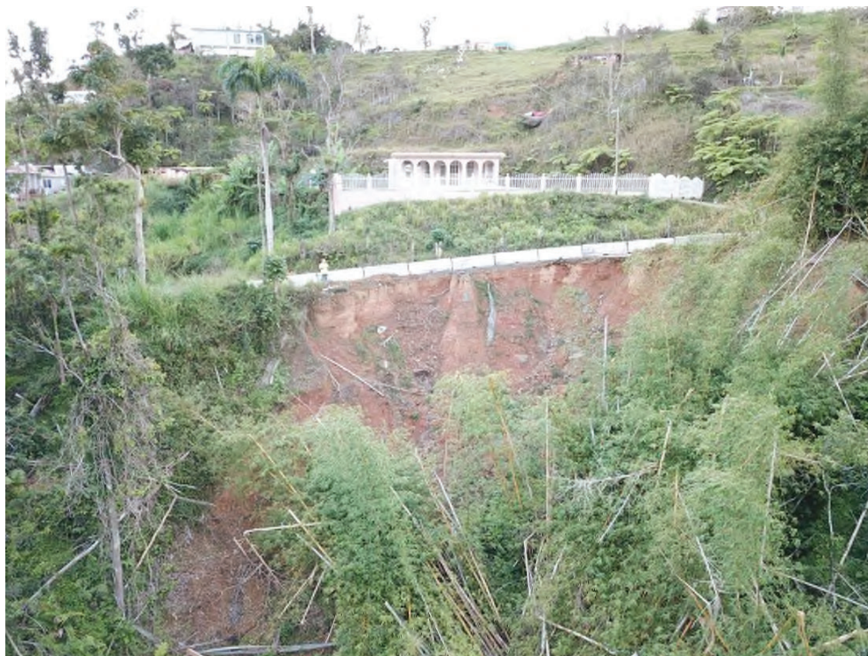
Figure 3: View of the Landslide at PR 179 Km 13.25 Approx.
