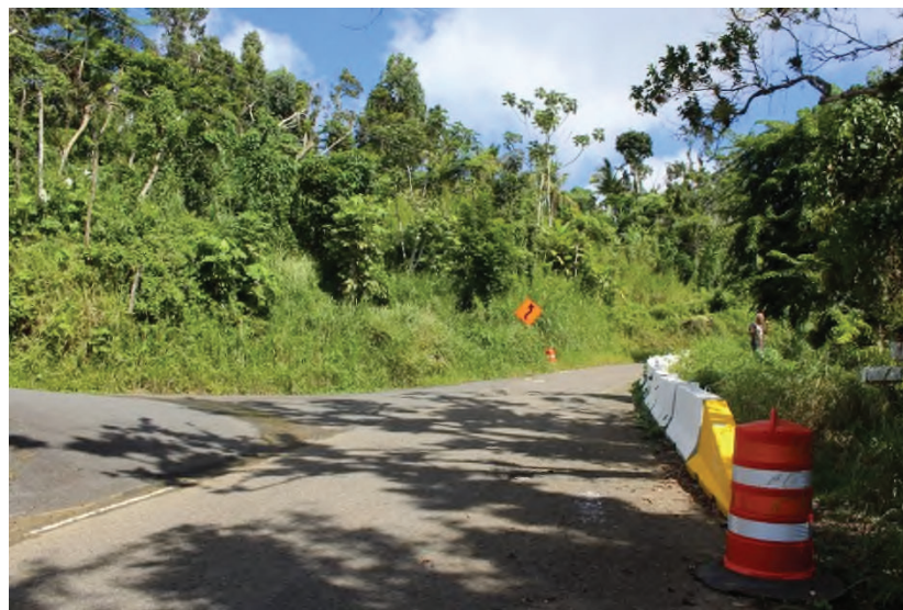
Figure 30: View of the Landslide at 13.25 from the South
