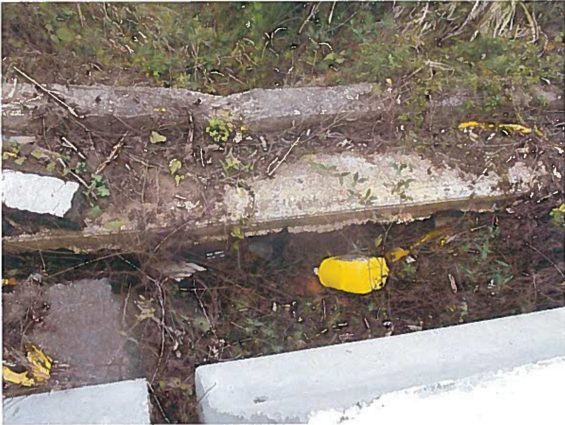
Figure 25: Photo 6 It Illustrates the Damage of the Collapse to the Curb of the Road.
