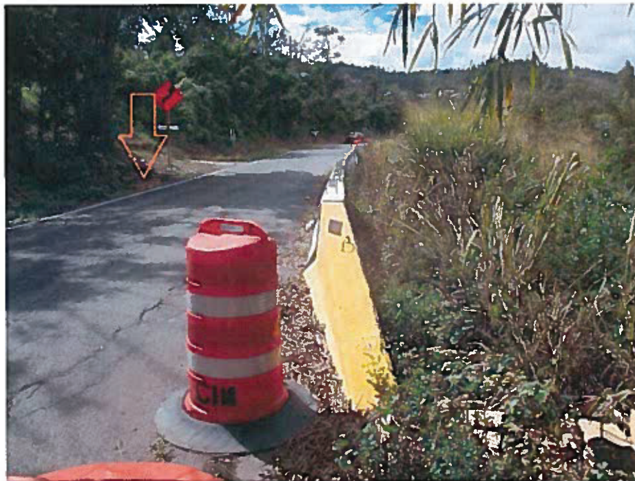
Figure 24: Photo 5 View Towards the Southwest of the Project. The Arrow Indicates the Place of the Storm Drain.
