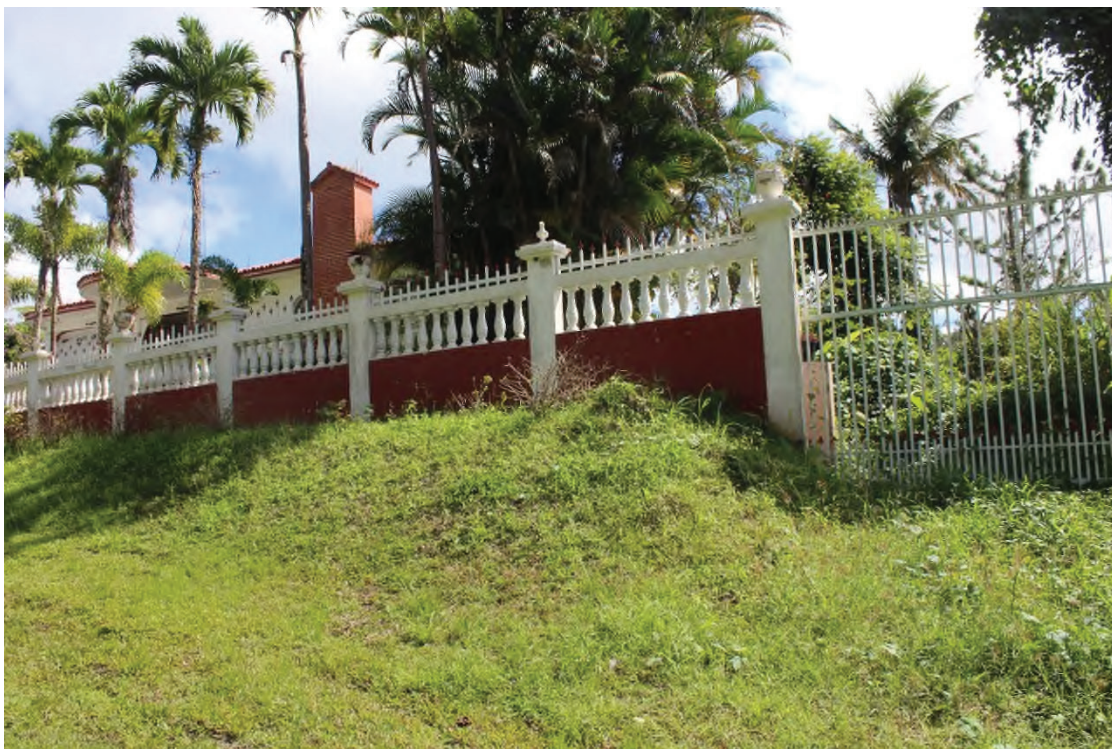
Figure 28: Area at the Side of the Road at km. 13. 35 Aprox. This Elevation is a Fill.
