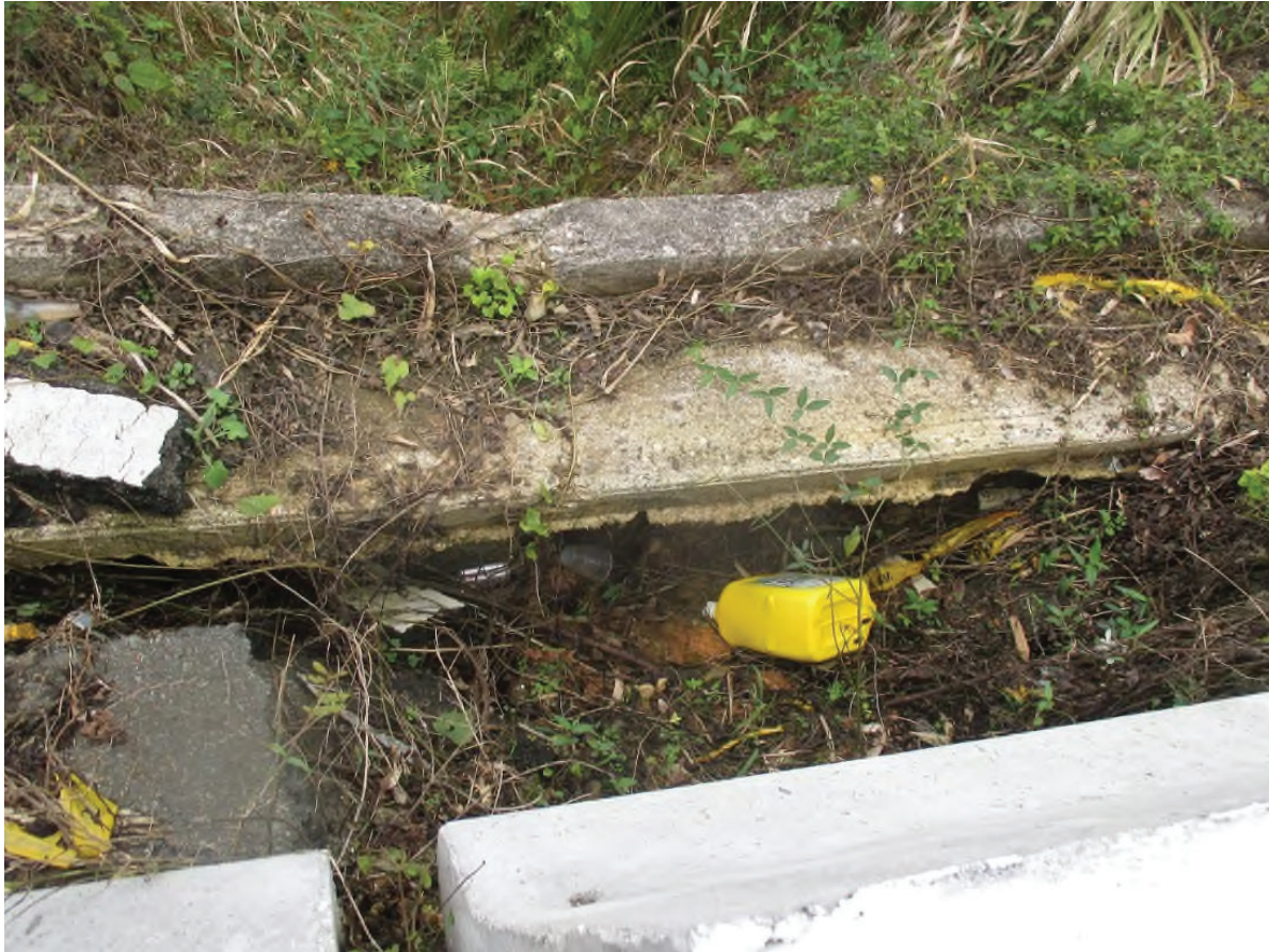
Figure 25: Photo 6 It Illustrates the Damage of the Collapse to the Curb of the Road.
